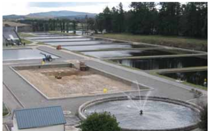
Cleaning a Traditional Slow Sand Filter (TSSF) at the Vartry Water Treatment Works, County Wicklow, Ireland (March 2009). Built in 1868 to supply Dublin City and environs.
